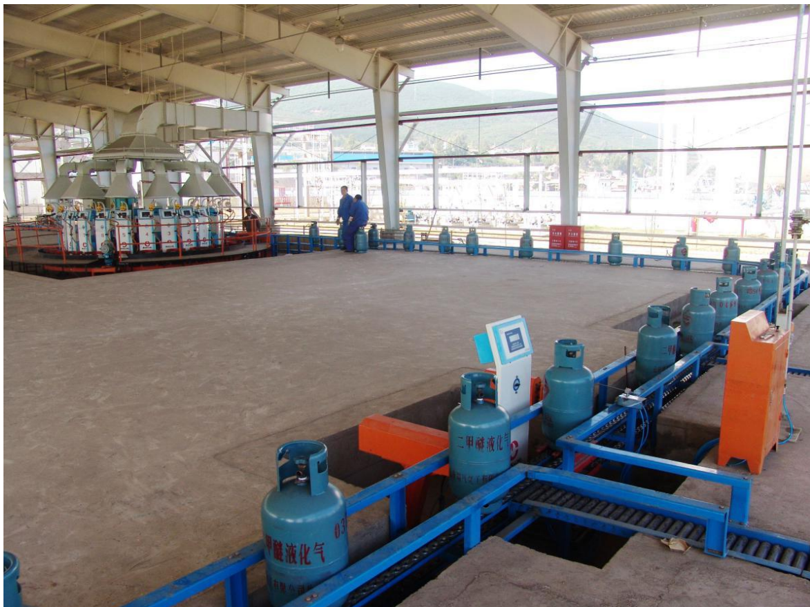
LPG cylinder Automatic Filling station
