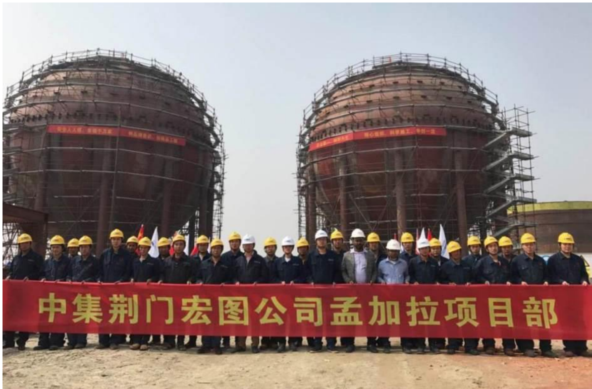
2x4000m 3 LPG tanks
